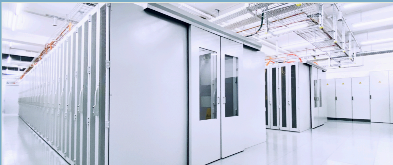
Ventilated customer racks (rear) with separate fiber and copper cable trays above. Central MMR/ODF racks (front).
